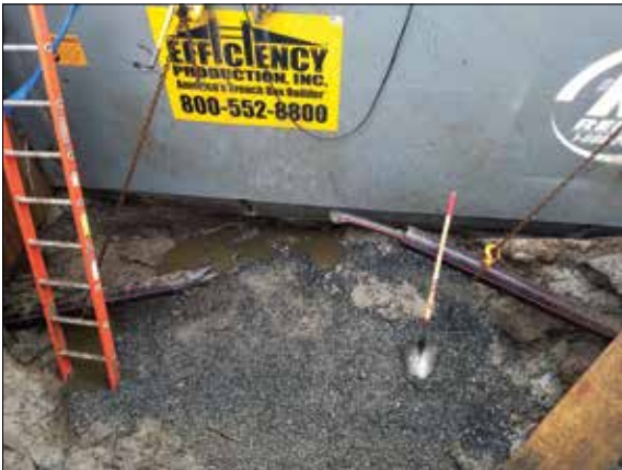
First damaged transmission line exposed
