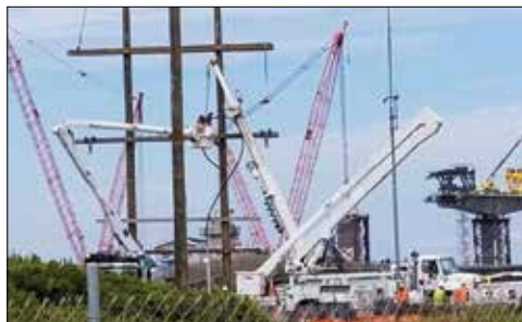
Ultimately, the overhead solution crossed the finish line first with transmission restored on August 3
