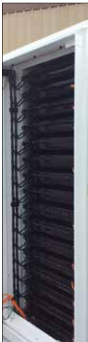
The installation consists of multiple Tesla batteries
