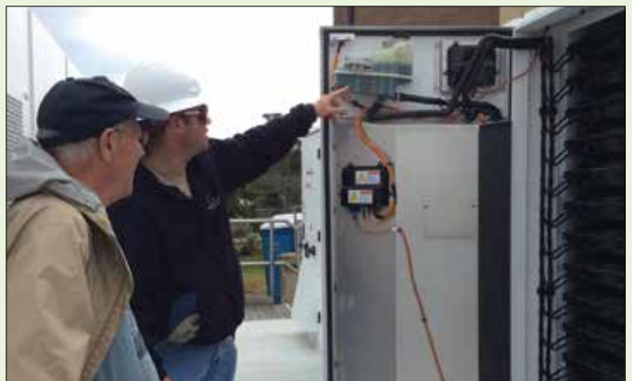
NCEMC's microgrid project manager Bob Beadle gives island reporters a look inside the Tesla installation.
