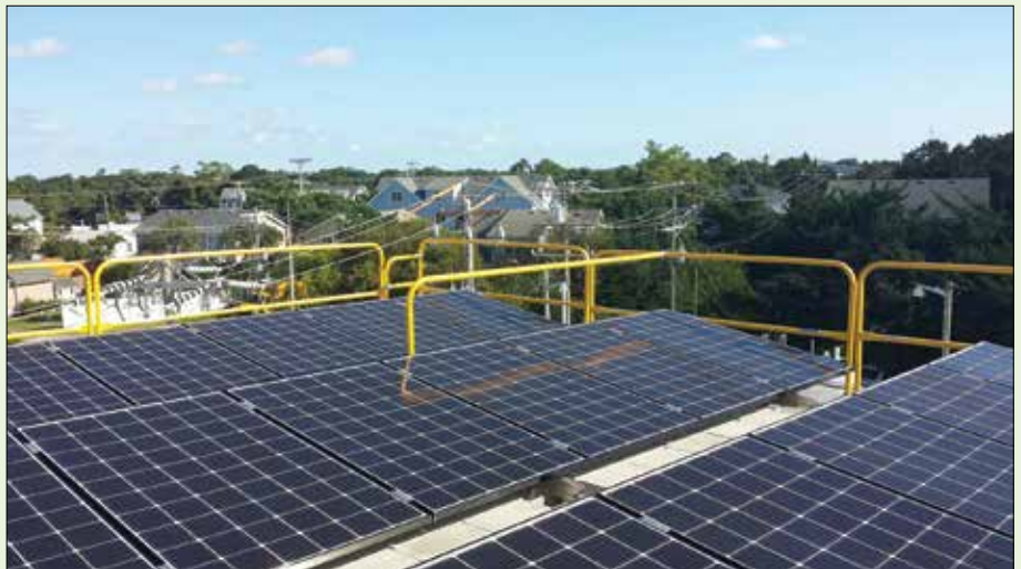
A 15 KW rooftop solar array was installed at the Ocracoke generating plant.
