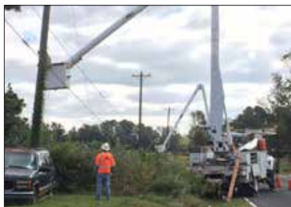
Merritt circuit damage
