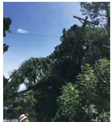
Tree damage at Boundary Canal knocked out service to the Engelhard substation (Photo by TW Allen)
