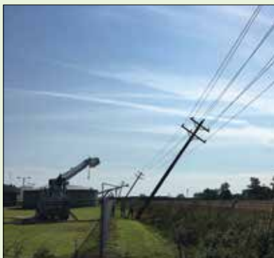
Crews straighten wind-sheared poles near the new Engelhard substation. (Photo by Adam Fyle)
