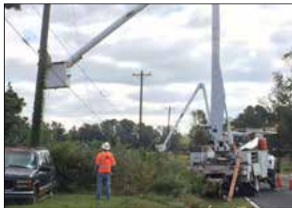
Merritt circuit damage
