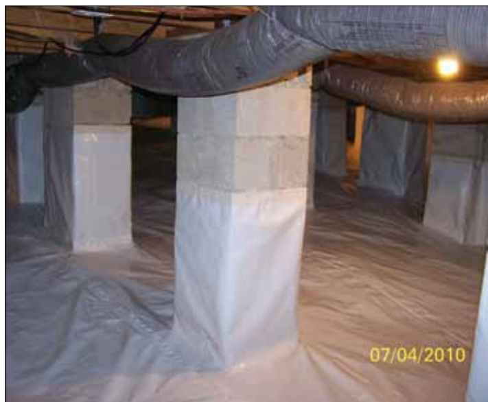
AFTER: A continuous, 8-mil vapor barrier has now been created with all seams sealed with an approved product (Larry Johnson photo)
