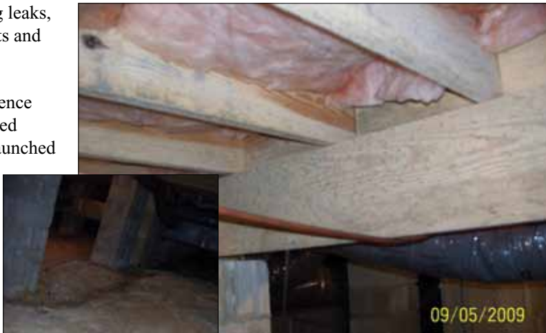
BEFORE: Mold and mildew appear on floor joists; No vapor barrier on the ground (Larry Johnson photos)
