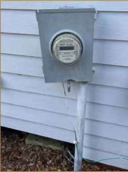
Meter base repairs required
