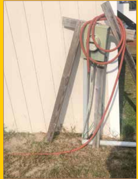
Meter base unstable; Unsafe placement of other items
