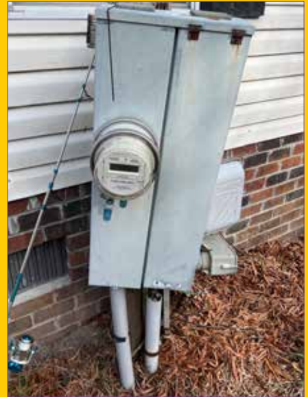
Meter base repairs required
