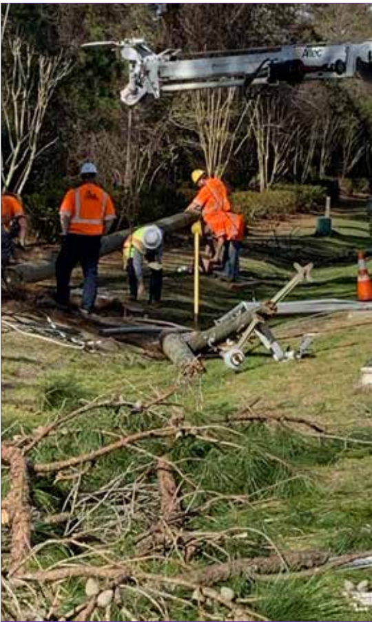
Contract crews assisted Tideland with wind storm repairs in Fairfield Harbour on February 7. Darren Bauer photo
