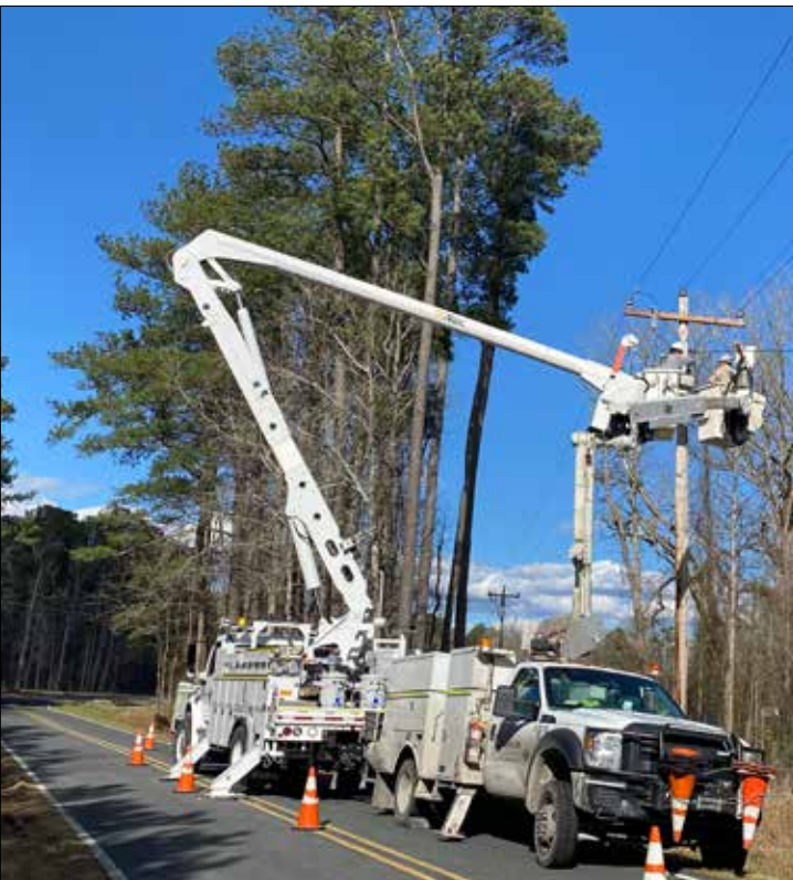
February 7 repairs on Ephesus Church Road in Blounts Creek. Wayne Brackin photo
