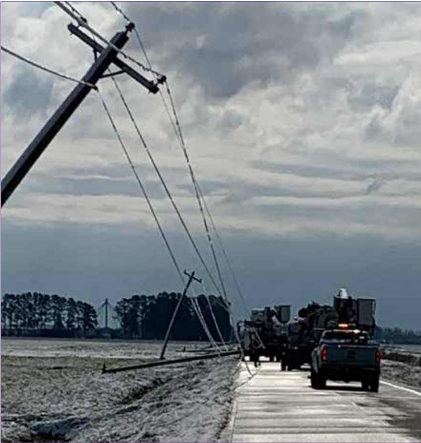
Lee Electric contract crews replace broken poles on Shirley Farm Road in Pinetown. Paul Spruill photo
