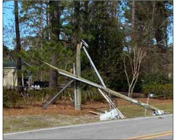
Distribution system damage at Fairfield Harbour on February 7. Timothy Ipock photo
