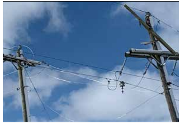
For every half-inch of ice on a distribution line, the result is one foot of sag.
