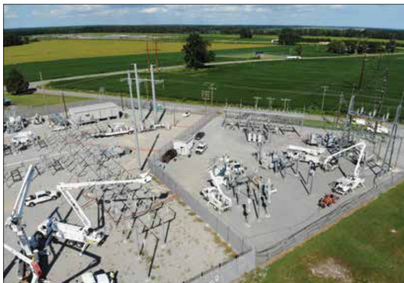
Crews from Tideland EMC and Dominion Energy worked jointly on the new transmission line connection at their respective Pantego substations. (Jim Chrisman photo)
