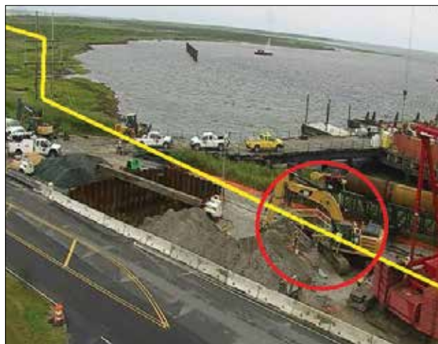
Yellow line depicts path of buried transmission line with red circle being point of impact. (Credit: Sam Walker, OBXVoice)
