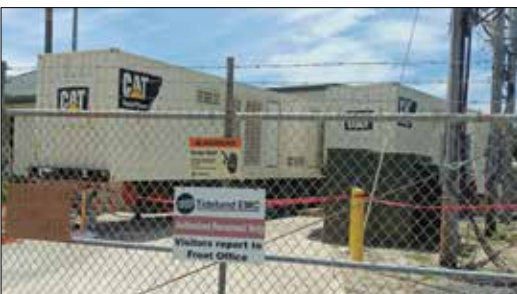
Three mobile generators provided electricity for Tideland's Ocracoke members
