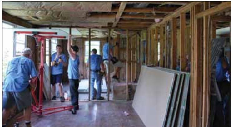
Crews lost a half day of work due to tropical storm Beryl
