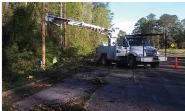
Tideland crews replaced 17 broken poles following the April 25 event. Photo: Kenneth Neal, Tideland EMC
