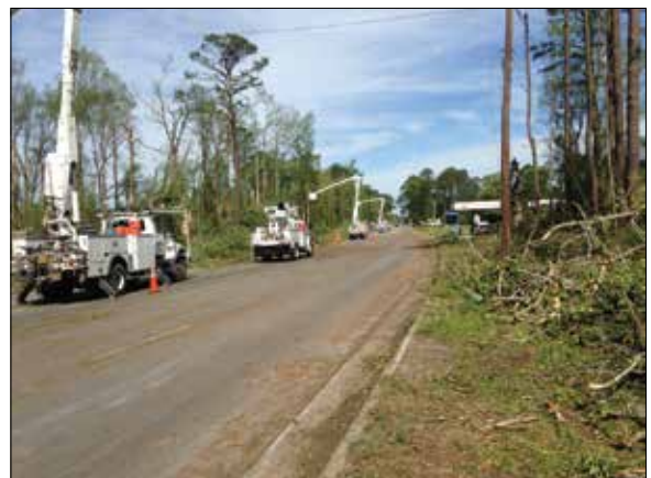
Co-op crews make repairs on River Road in Washington. Photo: Michael Marslender, Tideland EMC
