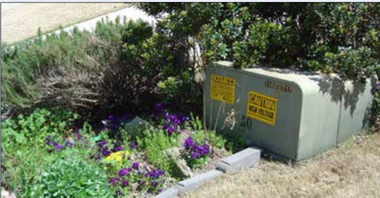
Never obstruct a padmount transformer with vegetation, decorative items or fencing. Remind children that these are energized pieces of utility equipment and are not appropriate for sitting on or using as a base for a game of tag.
