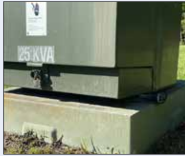
When a padmount lightning arrester operated at Camp Caroline, it became lodged between the cabinet and pad. Photo by Ryan Weston
