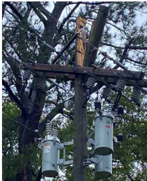
Replacement of a damaged joint-use pole necessitated a planned outage for 112 members east of the Y on River Road in Washington the night of September 23. Photo by Michael Marslender
