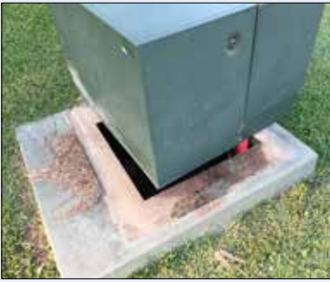
A transformer cabinet that floated out of position in Oriental. Photo by Edward Abrams
