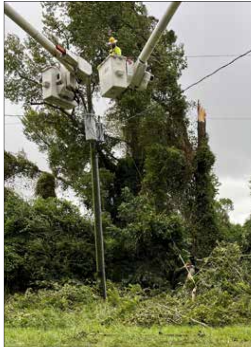
Contract crews with Lee Electrical work to restore power to members in the Yeatesville area of Beaufort County. Photo by Darren Bauer
