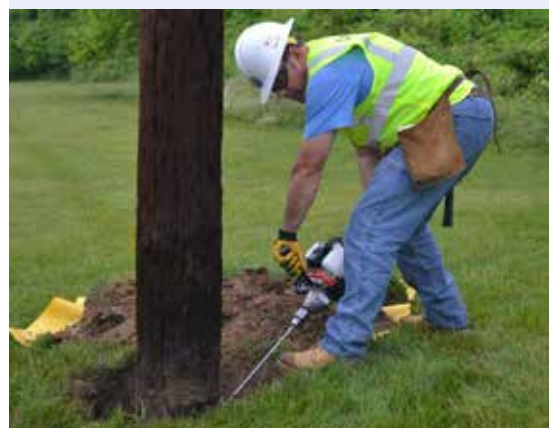
An Osmose contractor bores into a pole to inspect for internal signs of decay.
