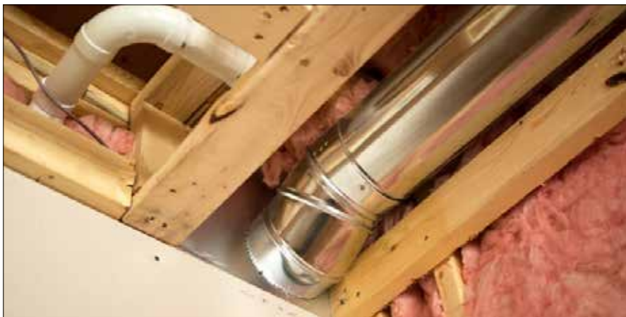
Placing ductwork in conditioned space can help reduce energy losses.
